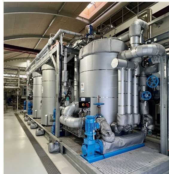
The Cambi THP system in operation at Damhusåen
