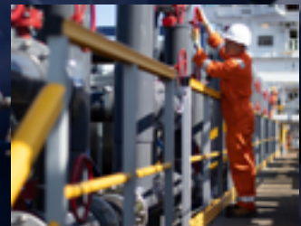
Technician adjusting the valve orientation on the CleanTreat® system
