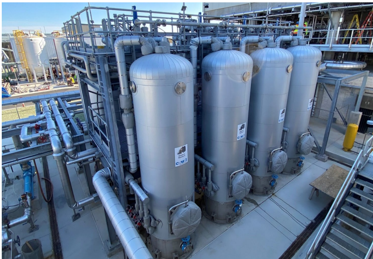
Photo: THP similar to the commercial scale systems planned at Secunda Operations (courtesy of Cambi)
