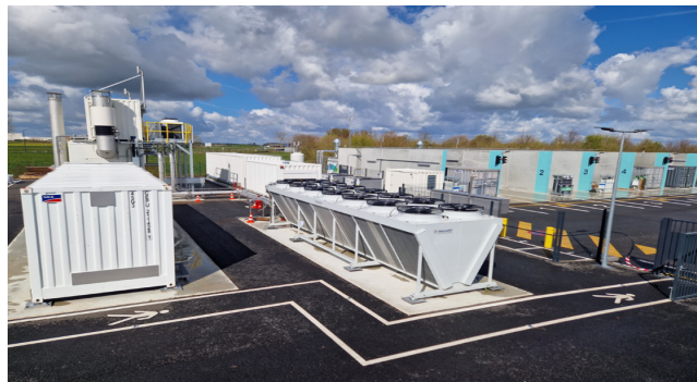
5 MW site at Croixrault, Hauts-de-France, France
