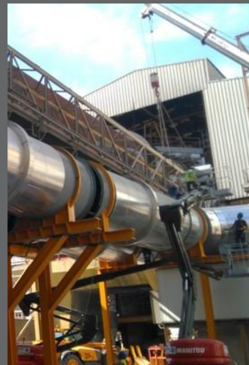
THERMAL SUBSTITUTION IN SOUSELAS
